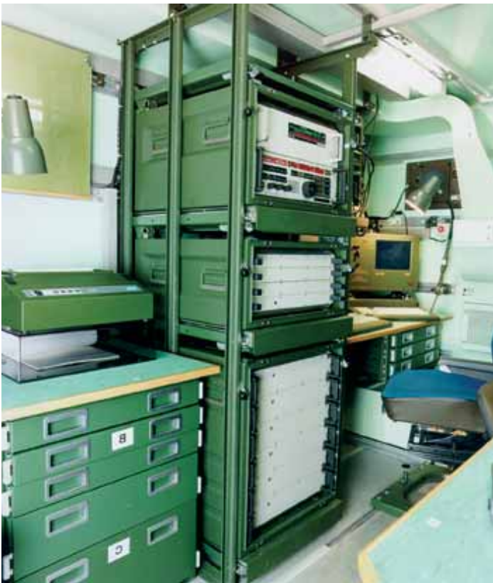
Semi-mobile radio station with several transceivers, supplied from 24 VDC on-board power supply
